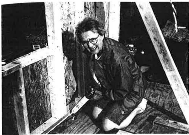
Figure 1 Thorough air sealing, while labor intensive, does not require skilled workers and can easily be done by volunteers.
