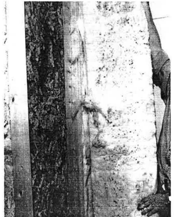
Figure 10 Surface of unfaced R-13 batt insulation showing evenly distributed fungal growth.
