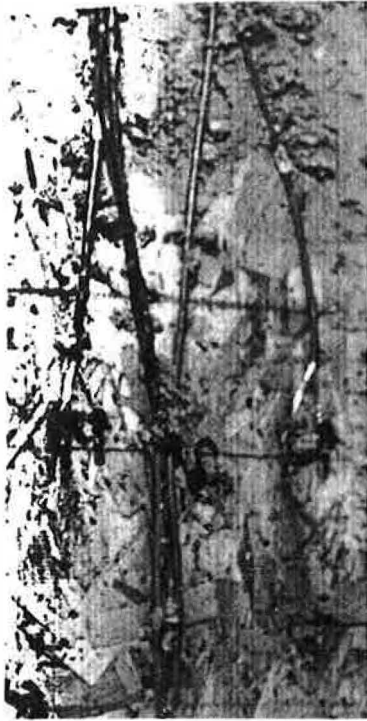
Figure 11 Rust on metal fasteners in cellulose cavity without vapor diffusion protection.
