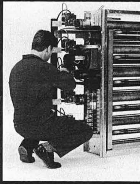
Direct gas-fired heaters in air-handling plant for a new Tesco store will provide major energy savings compared with LPHW systems.
