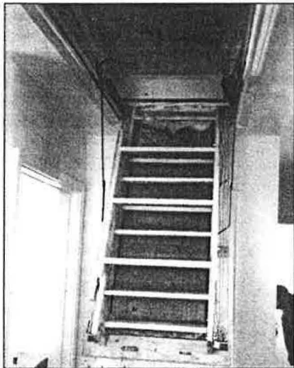
The pull-down stair is insulated, in order to maintain the R-value of the attic insulation.
