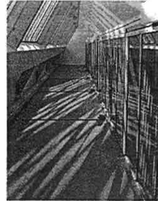
figure 24 : air extraction duct
