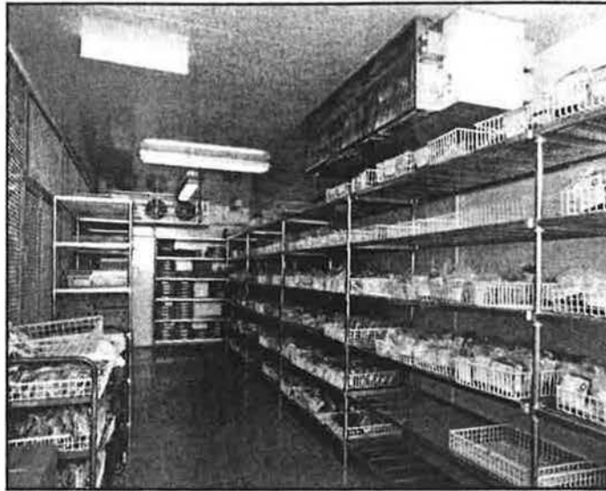
This cold room by Lindsell Dewell is at the Colindale premises of the North London Blood Transfusion Centre
