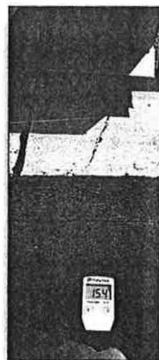
FIGURE 3. Non-contact infrared thermometer taking a surface reading of the roof surface below an outdoor air intake. Note the high temperature (154 F) for energy efficiency implications of such conditions. See the related article on economizer optimization on page 35 of this issue.
