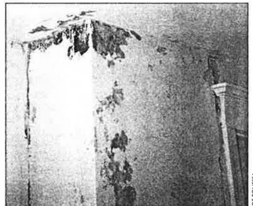
Wall damage that had appeared on the second floor around the chimney gradually worsened over time. It would reappear, even after the new roof was put on.
