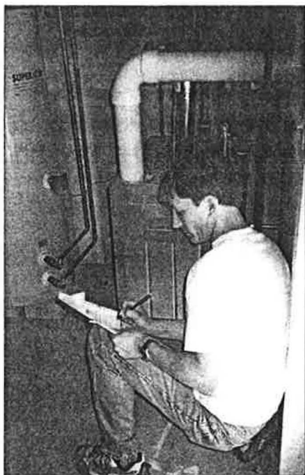
Home energy rater Pat Haller, of the Vermont Investment Corporation, checks the efficiency of this furnace and water heater.
