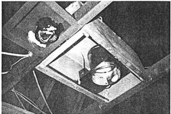
Figure 3 — Looking up into the roof of one of Lentz's new homes, we see the careful attention given to air sealing. The airtight box for the recessed light fixture is made of 1-inch-thick pieces of scrap foam assembled with tape and expanding foam. Lentz says he likes to leave plenty of air around the light to prevent overheating. He says that none of his houses have ever experienced the "blinking light syndrome," indicative of overheating. The Lessco airtight electrical box to the left is for a hard-wired smoke detector.
