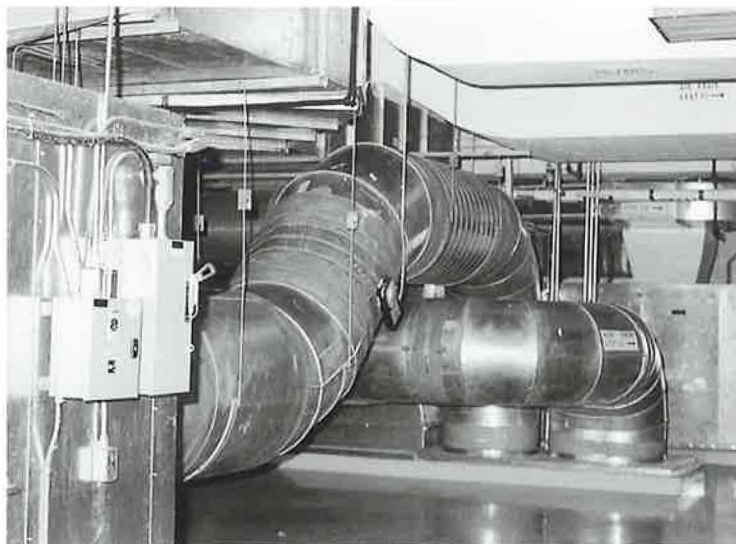
Figure 2: Dual duct system at the Canadian Space Agency.
