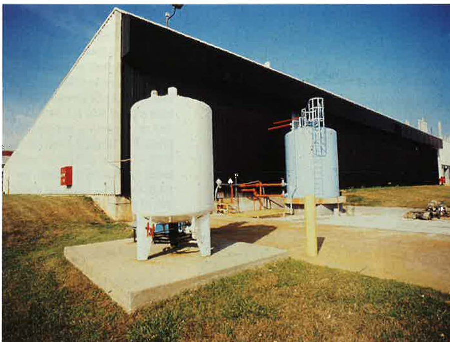
Solarwall at GM Battery Plant.
