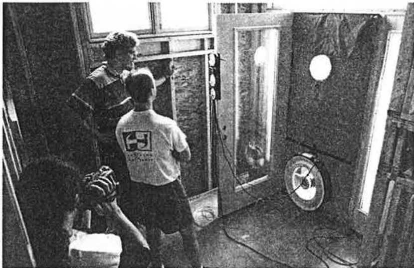
Field commissioning tests prior to wallboard installation at the Washington's Landing home identified thermal shell and duct system weaknesses at a time when modifications were most cost-effective. Pre-drywall tests demonstrated 0.13 ACH.
