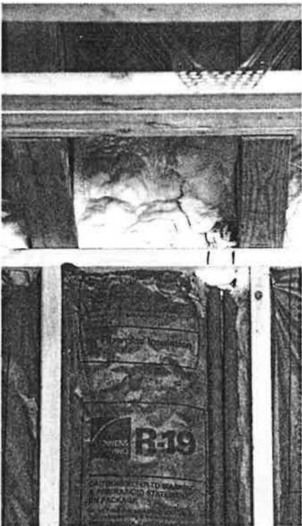
Icynene spray-in flexible foam insulation was used at Washington's Landing in areas where insulating with more traditional materials was difficult. Here, the foam is sprayed into the band joist area, with fiberglass batt insulation used in the wall cavity below.
