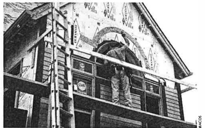
For this house at the Village at Washington's Landing, in Pittsburg, Pennsylvania, builder Montgomery & Rust specified Wverzait composite wood and resin siding, which features excellent moisture resistance. Rigid foam joints were taped to minimize air infiltration.
