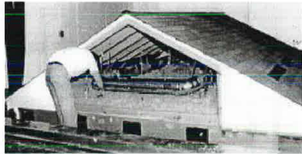
Figure 3 Photograph of the residential attic test section with the uninsulated attic duct system suspended from the rafters.
