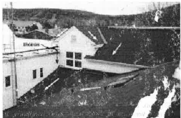
Figure 11 Roof surfaces that drain valley over dispatch center.
