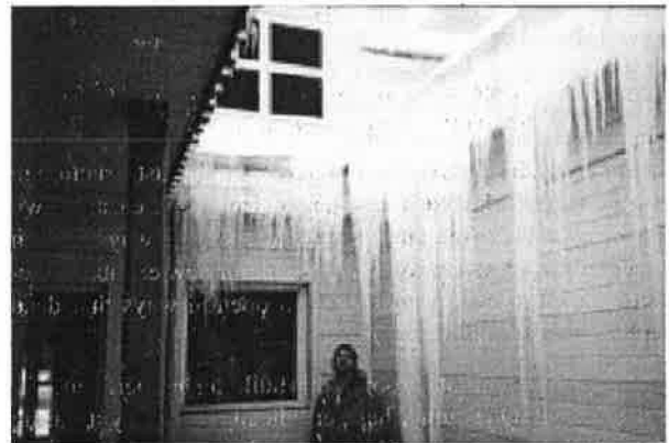
Figure 10 Icings and ice dam at eaves of problematic valley over dispatch center. Icicles in the valley were removed, the day before this picture was taken.
