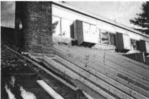
Figure 6 Notches in 2x6's allow cross-ventilation, at chimney and at large building exhaust hoods. Exhaust structure shown in Figure 5, not altered.
