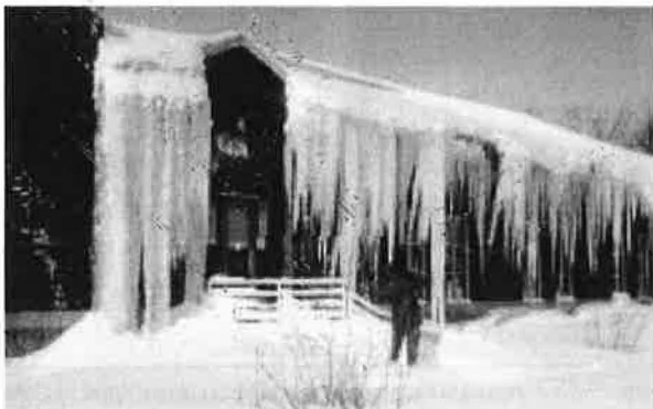
Figure 2. Severe problematic icings developed all along the eaves of this dining facility.
