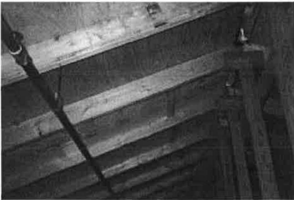
Figure 15 Extruded polystyrene insulation added to the underside of a portion of the original roof deck.
