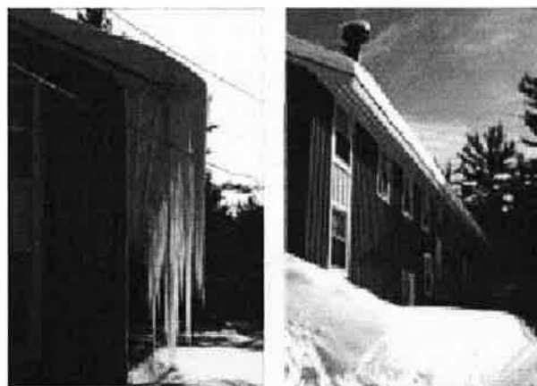
Figure 1 Two identically constructed roofs photographed at the same time. The building on the right, with no icings, was unheated.
