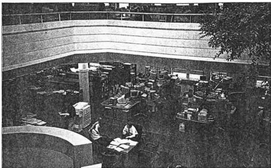
The ground floor offices at Co-operative Retail Services, viewed from an atrium. Due to the unreliable lighting control system, the metal halide uplighters tend to be on outside of normal office hours, contributing to an 'uplift' of 3-4°C to the supply air temperature in the first floor plenum.
