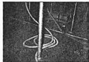
Lighting ballasts in the floor plenum are believed to be responsible for a 1°C hike in supply air temperature.
