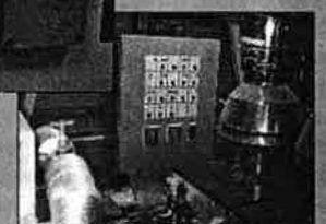
...but thumbs down for placing the summer/winter switch at the end of a plantroom obstacle course
