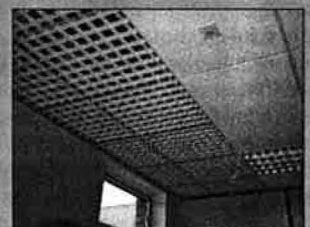
The perforated ceiling has caused some cross-talk problems.
