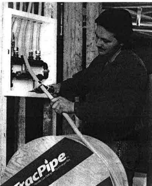
Figure 4 — CSST is installed to a service panel with central manifold.
