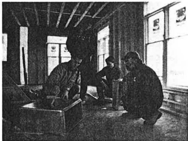
Figure 3 — On-site training helped familiarize the HVAC crew with Owens Corning's EnDuraCoat fiberglass duct board.
