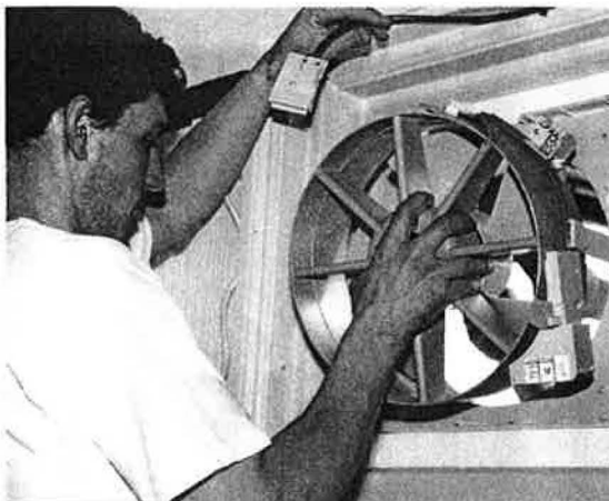
Replacing the extract fans proved relatively straightforward despite the fact that the pub is a Listed building.
