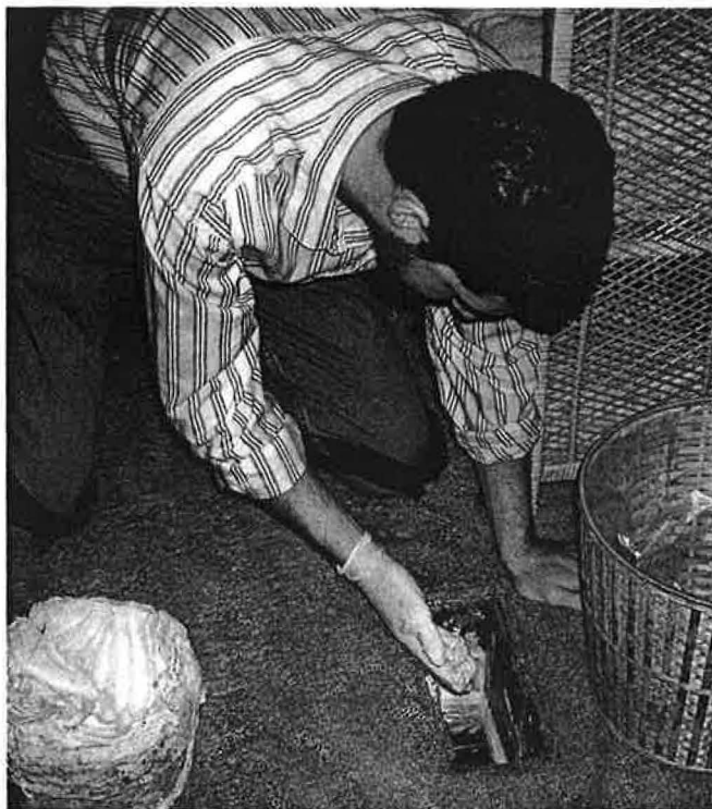
Sam Karp of Delta-T seals a register boot after measuring initial leakage.
