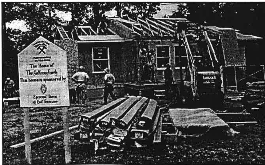
Figure 3. Habitat for Humanity's 1997 Jimmy Carter Work Project provided a good test for the effectiveness of checklists and instructions in making a first step at improving energy efficiency in affordable housing.
