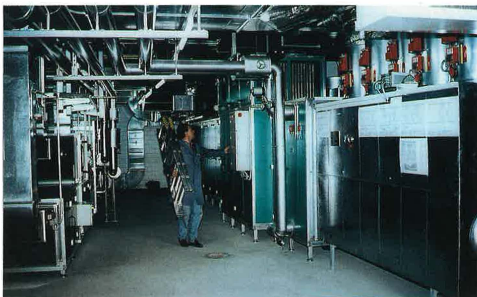
Ventilation plant with air recycling.
