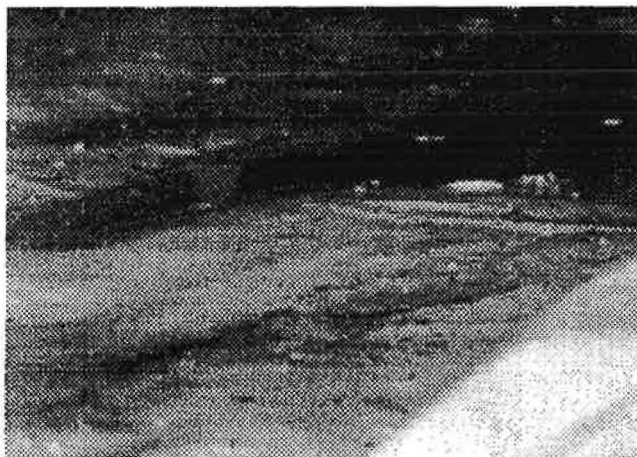
Figure 3 Water on vapor barrier
