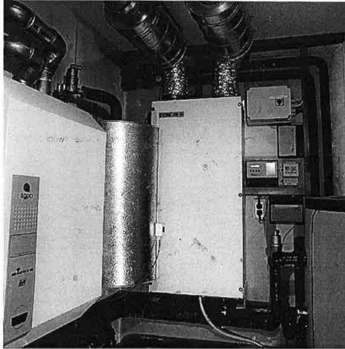
Figure 4 View in the technical room
