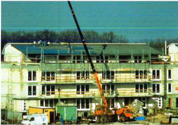
ROOF-INTEGRATED COLLECTORS ON A MULTIFAMILY BUILDING IN NECKARSULM, GERMANY
