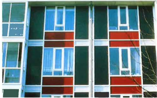
FACADE-INTEGRATED SOLAR COLLECTORS AND GLAZED BALCONIES
