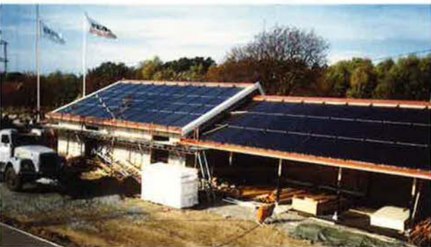
ROOF MODULE COLLECTORS IN ONSALA, SWEDEN
