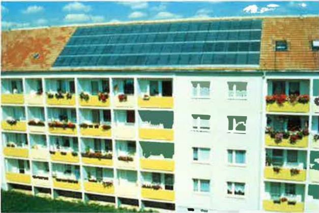
ROOF-INTEGRATED (MODULE) COLLECTORS ON A MULTIFAMILY BUILDING IN OEDERAN, GERMANY
