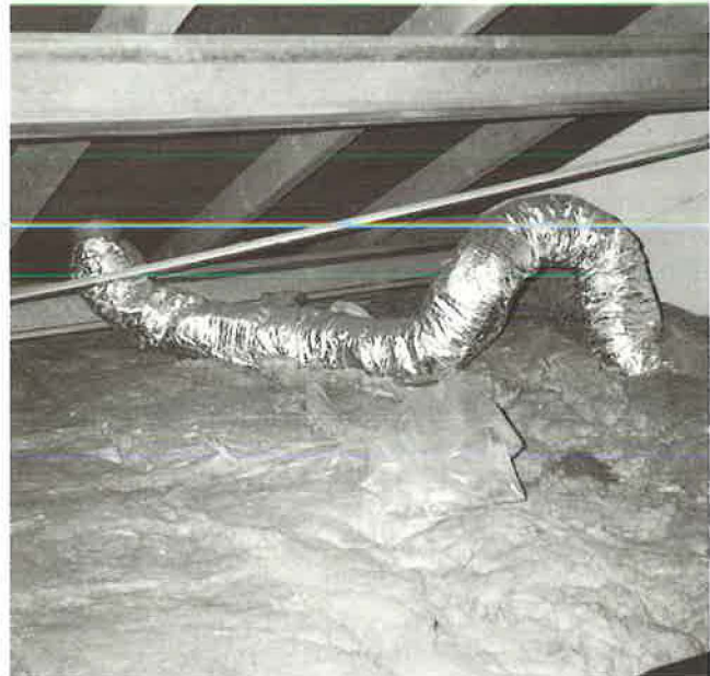
Figure 4 Badly installed flexible ducts with excessive length of duct work and tight bends
