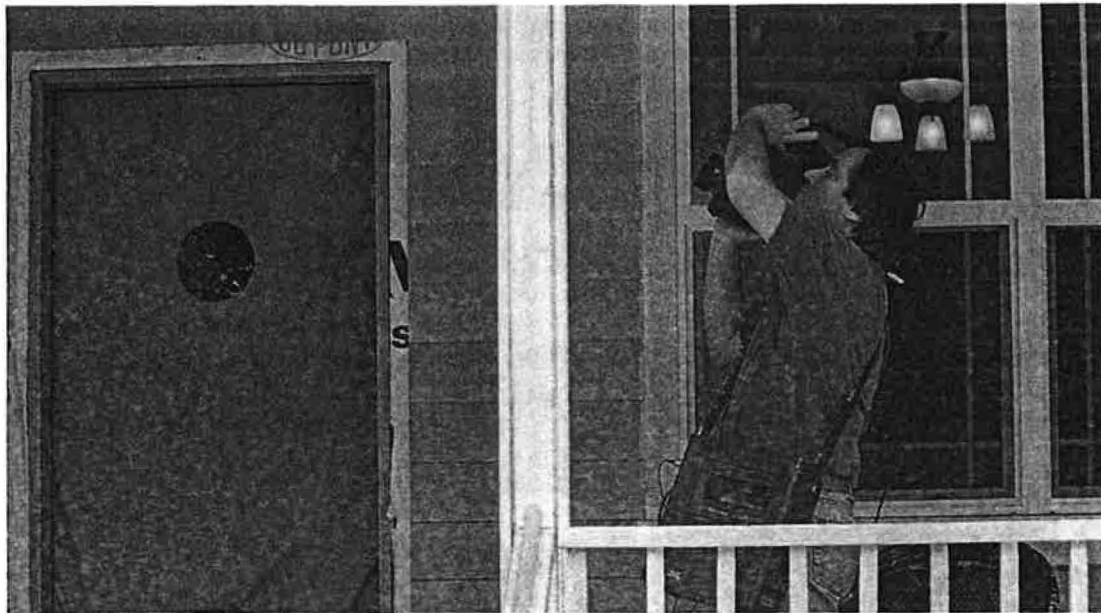
Filming the home with an infrared camera when it is depressurized illustrates where air is moving into and out of the home, and the path it takes.
