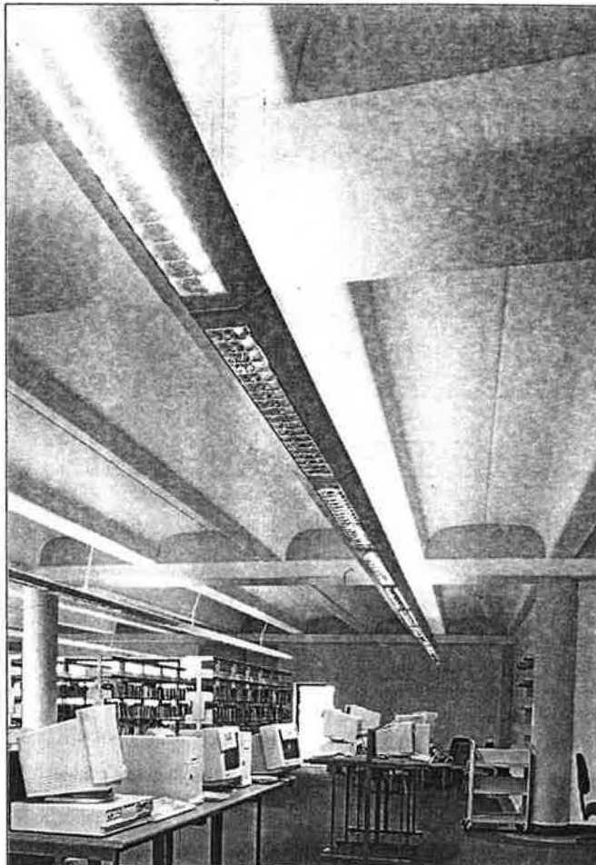
Category 2 luminaires suspended from the coffered ceiling at 3.6 m centres provide 350 lux on the working plane in the main occupied areas.
