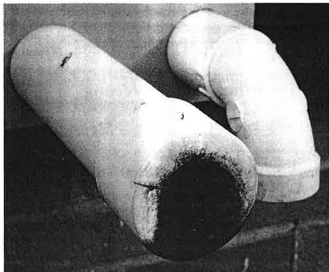
Soot is visible on this outdoor furnace outlet where concentrations exceeded 4,500 ppm (the maximum reading on our test instruments).
