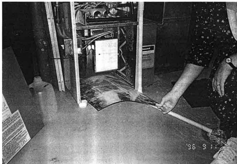
This new furnace has an open bottom section covered with a plate, which the installers failed to attach properly. The unsecured plate warped and allowed air to leak into the furnace from the basement, instead of being pulled through the electronic air filter and return duct on the right side of the furnace.
