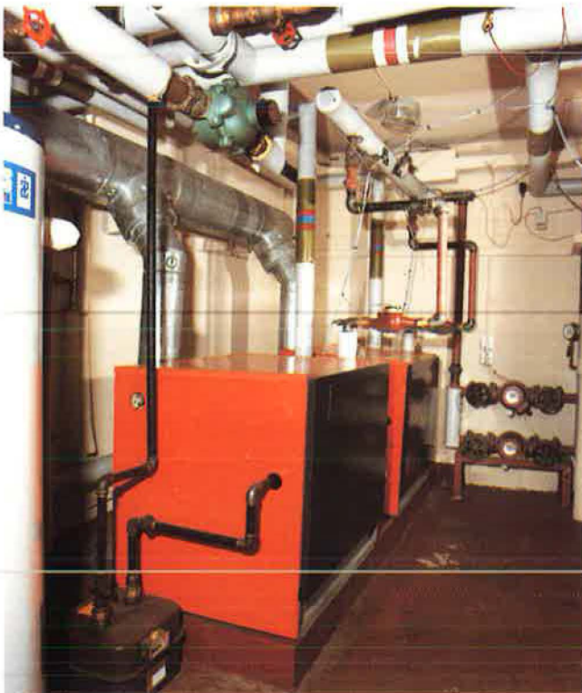
Broag boilers in Holly Court boiler room.
