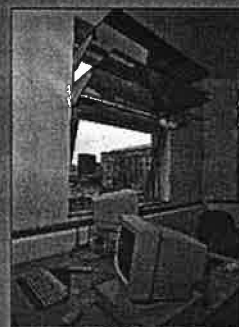
At APU, the twin internal light slates of semi-transparent reflective glass have proved ineffective in enhancing light levels deep into the space, as the daylight is reflected into the coffers of the waffle slab ceiling.
