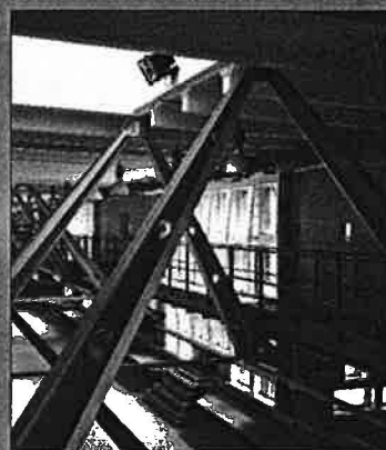
De Montfort: the striking characteristics of the high-bay SON lamps do not encourage frequent manual switching.
