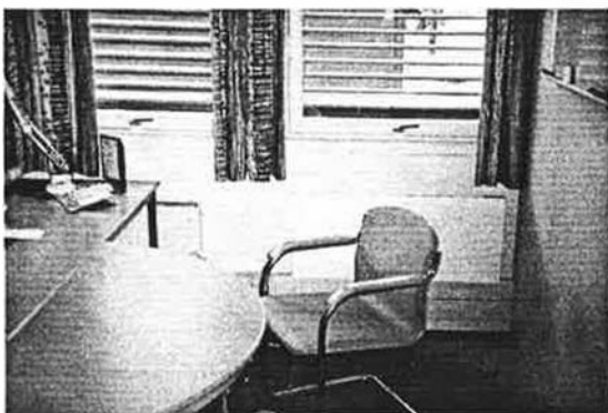
Panel ovens for heating in cellular offices. The ventilation air inlets are located behind the panel ovens to ensure preheating. The inlets are designed to give sound attenuation
