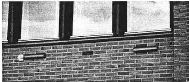
External ventilation inlets
