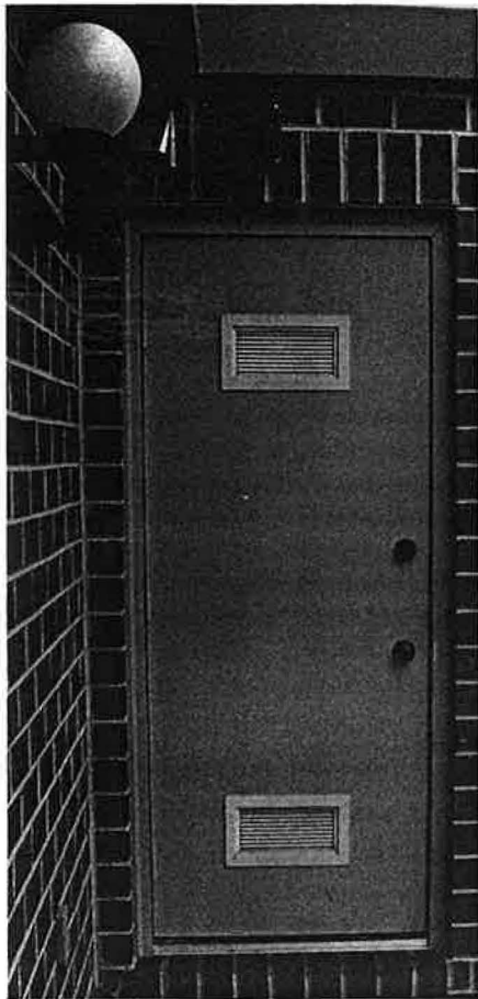
Combustion air inlets in the door to the mechanical room. The existence of these intentional openings and a supply duct on the furnace plenum combined to produce significant house depressurization during the blower cycle.
