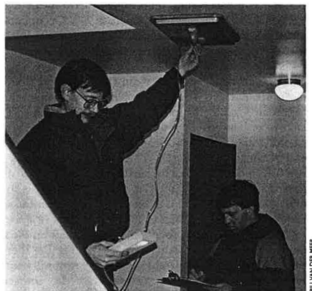
Pressure pan testing revealed significant leakage to the outside. Since the ducts were contained within the building envelope, most of the leakage was attributed to a register supplying heated air to the mechanical room.
