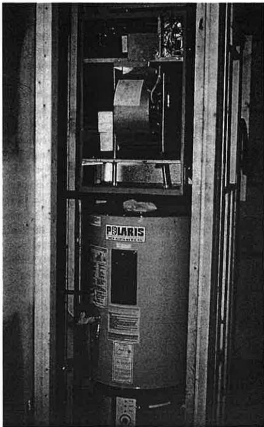
In 64 of the rehabbed units, the contractors installed combination heating systems (made up of a water heater with a fan coil) that meet both space and domestic water heating needs.
