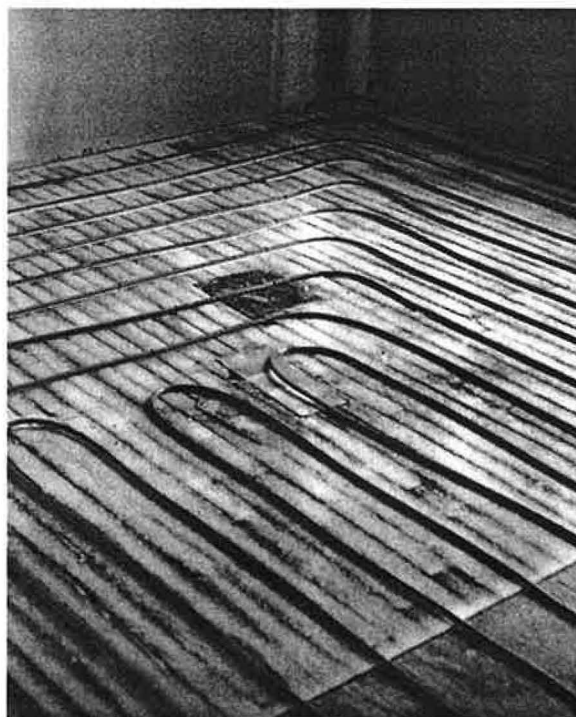
In one 10-unit building the contractors had a chance to install a radiant floor heating system. The building floors were in such bad shape that plans called to level them with lightweight concrete, so the contractors installed the radiant system's plastic tubing over the existing floors before adding the concrete. This method saved $10,000 in first costs over installing baseboards, and the building is both comfortable and efficient.
