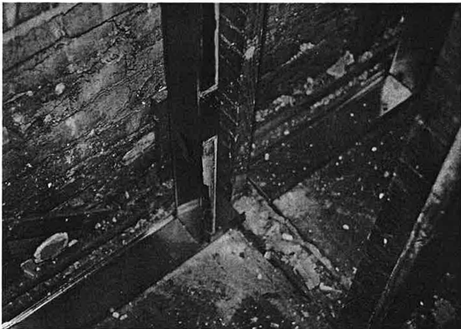
Since the masonry wall surface is usually rough and uneven, the contractor holds the studs back about 1 or 1 1/2 inches from the walls to produce a straighter frame. This also leaves a deep framing cavity, which can accommodate more insulation.
