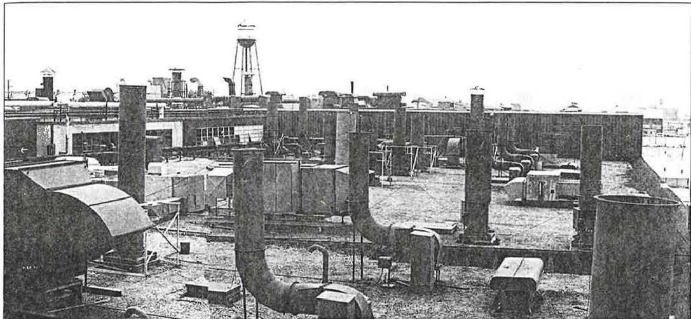
HVAC engineers are often confronted with 'a forest of fans' when asked to correct a ventilation problem for an industrial client.
