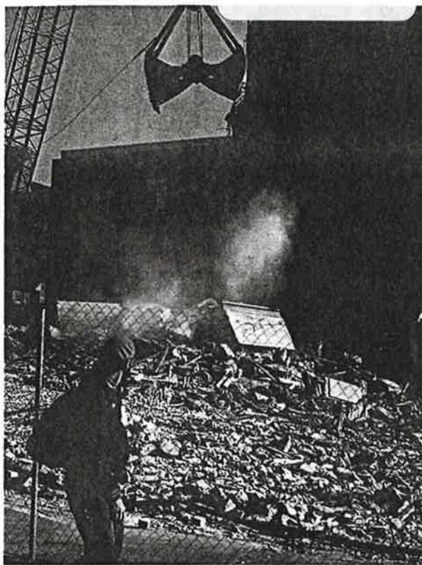
Airborne particles are generated at construction sites by processes such as demolition, excavation, grinding and sanding. Containment strategies are predicated on the potential impact to construction workers and building occupants.
