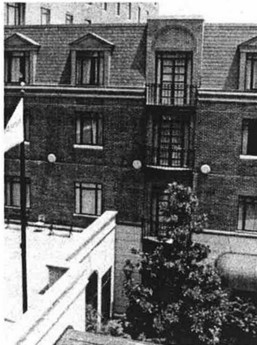
Figure 1-6. Rainwater leaks masked a significant secondary source of IAQ problems at this luxury hotel, which developed severe moisture and mildew problems shortly after it was built.
