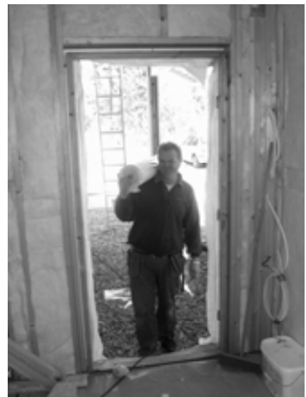
A very contented carpenter, after having received the 0.8 ach/h result, here carrying in the first roll of vapor barrier
