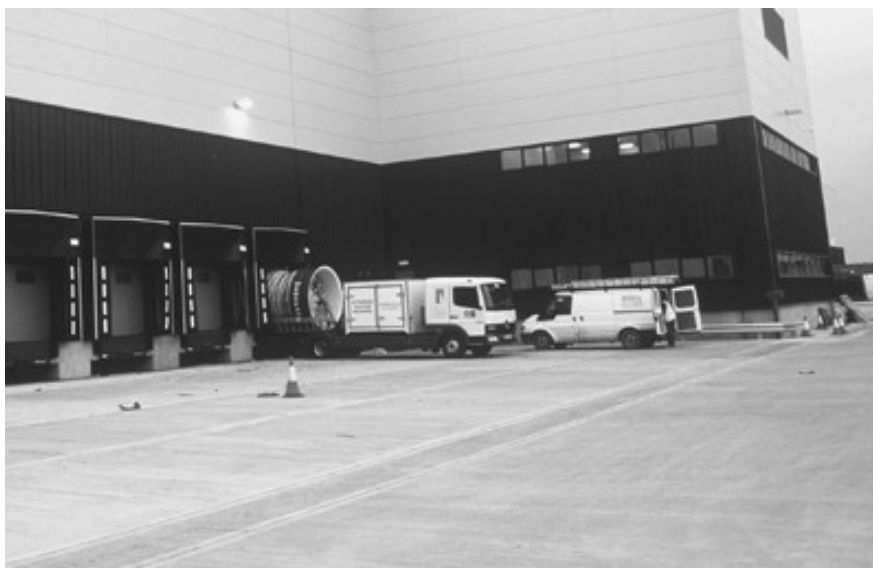
The Megafan positioned in a loading bay
