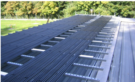
Figure 5: Unglazed collector mounted on the roof.
