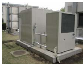
Photo 2 Water tanks and auxiliary heat source
