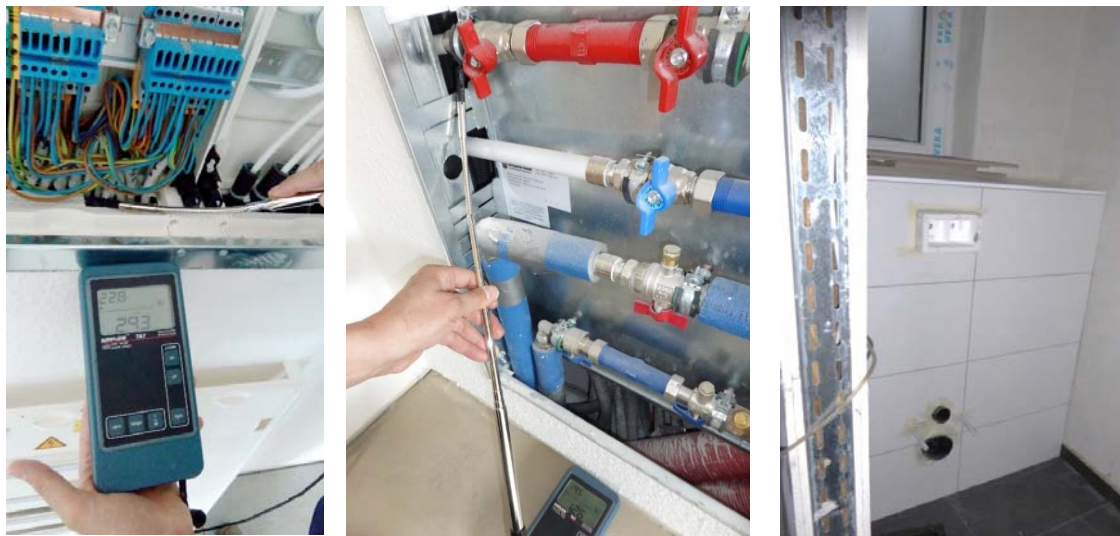
Figure 5: building IH : internal leakages were found in power distribution units, central water distribution units, pre-wall sanitary installation and internal partitions
