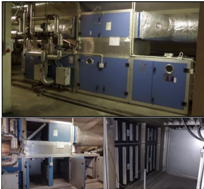
Figure 4 HVAC unit used for the natural ageing of the filters.
