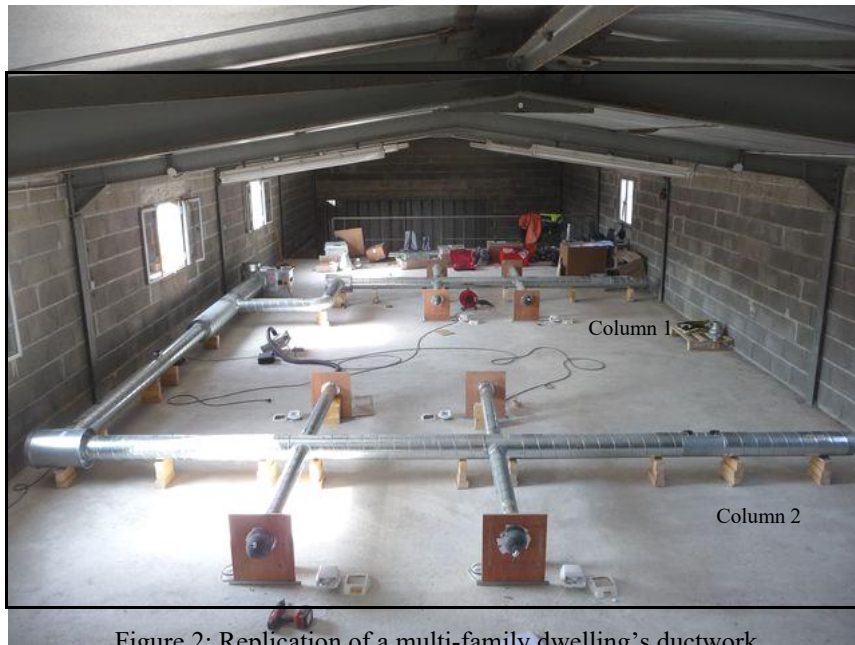
Figure 2: Replication of a multi-family dwelling's ductwork
