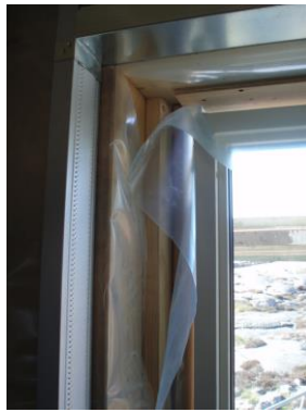
Figure 2: Window setting with two separate foils that will be sealed together to an airtight joint (Wahlgren, 2010).
