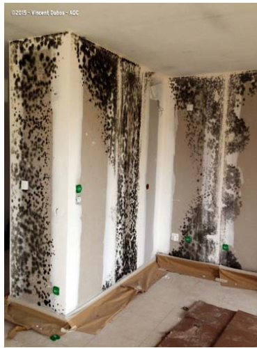
Figure 2 – Mould growth on drywall during the construction phase
