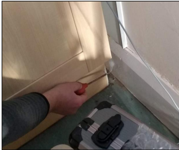
Figure 3. Photograph of the smoke pen survey, showing significant air leakage behind the kitchen cupboard.
