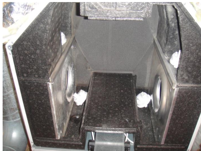
Figure 4: Example of temperature logger placement for the first measurement campaign. The heat-exchanger has been removed to place the sensors
