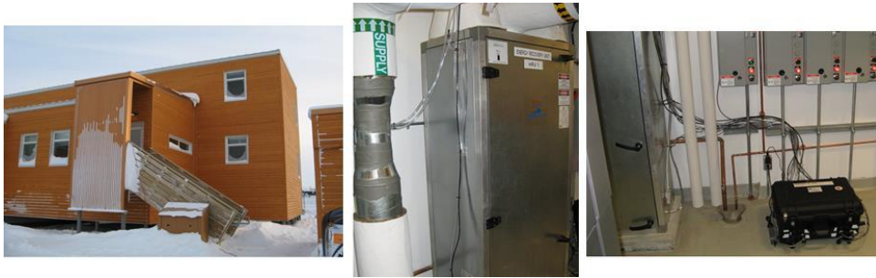
Figure 3. Triplex and deployed dual core ERV on CHARS campus in Cambridge Bay, NU
